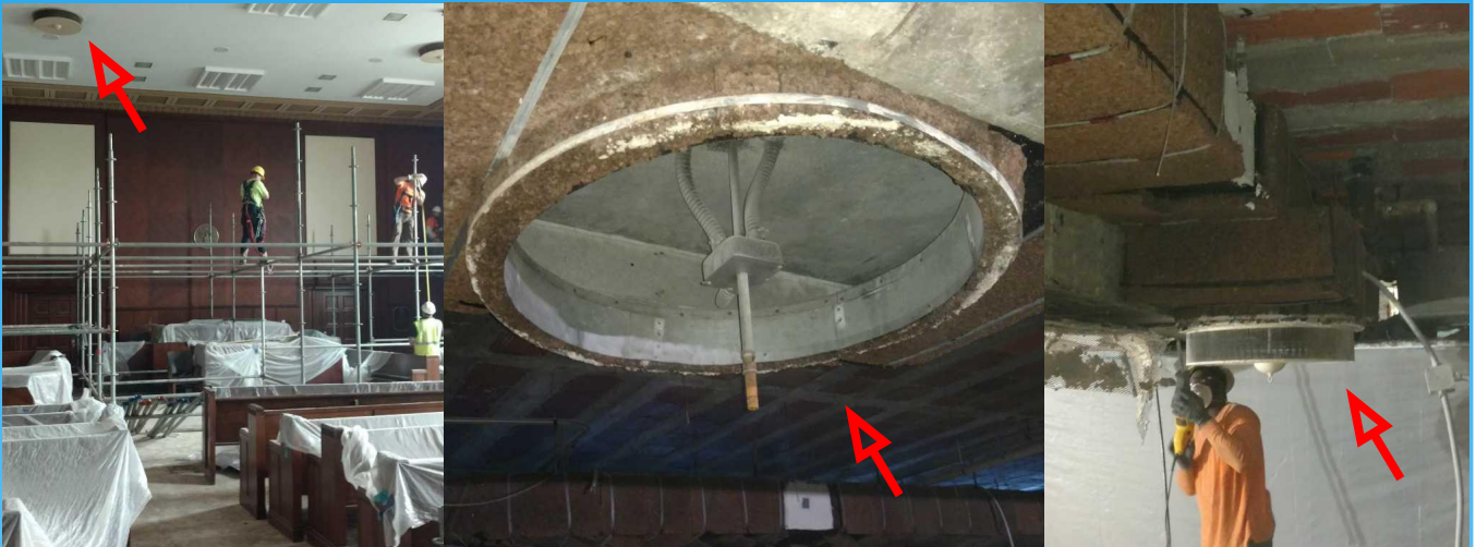
Scaffold erection in the ceremonial courtroom (left), worker standing on scaffold cutting ductwork loose (right), and original round supply air duct opening (middle)
